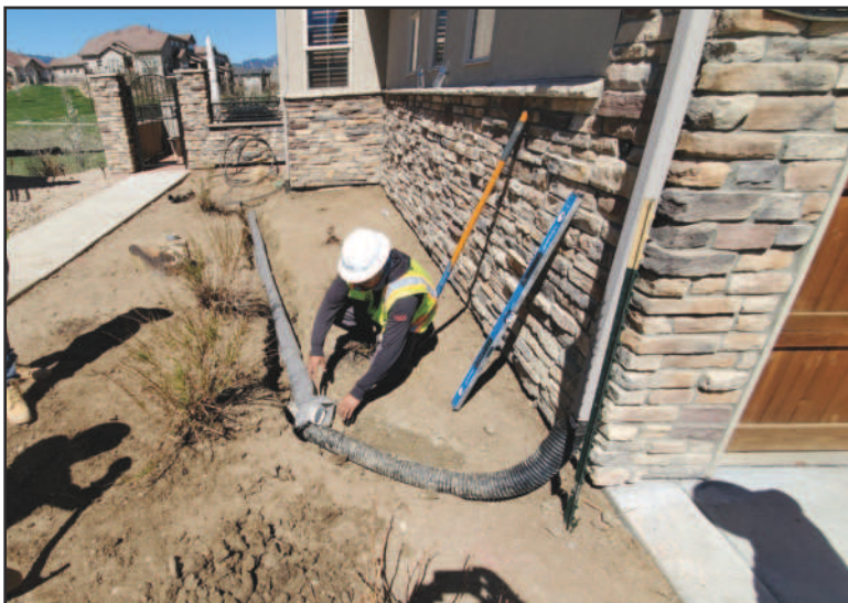
The crew is installing drainage systems to move water away from the foundation.
