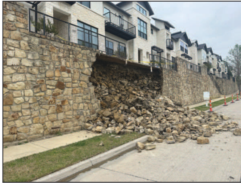
Emergency shoring was required on this soil bank and retaining wall.
