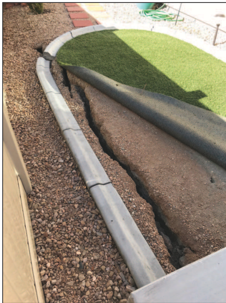
Signs of soil movement can be seen near a home foundation.
